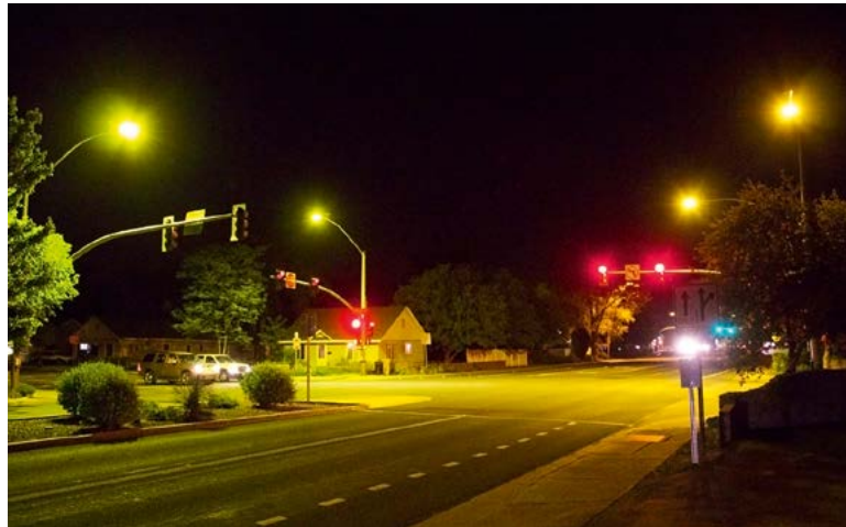
Figure 3: Filtered LED (left) and phosphor-converted amber LED (right) are shown here in a test installation at an intersection in Flagstaff, Arizona. The City of Flagstaff is currently testing these and other low-blue-light LED technologies for the replacement of its existing sodium municipal lighting system (credit: IDA / John Barentine)
