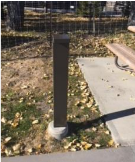
Figure 1. Dark sky compliant light post installed along the walkway to the new seawall and Peace Park exhibit in Waterton Lakes National Park.
